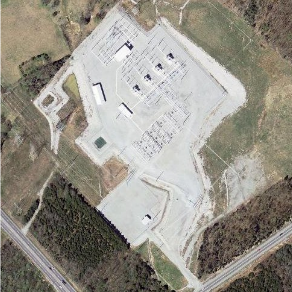
Figure 2-12. Aerial View of Typical 500-kV Substation
