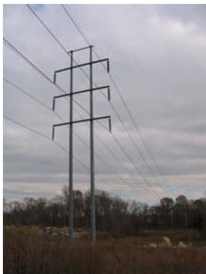
Figure 2-16. Double-Circuit Transmission Line, H-Frame 161-kV Transmission Structure
