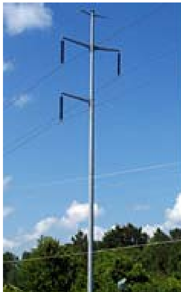
Figure 2-15. Single-Pole 161-kV Transmission Structure
