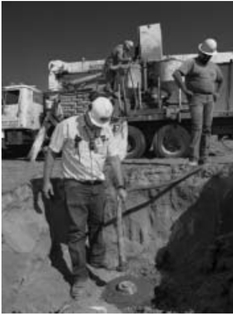
A well decommissioning crew places a brass marker on top of a decommissioned well.
