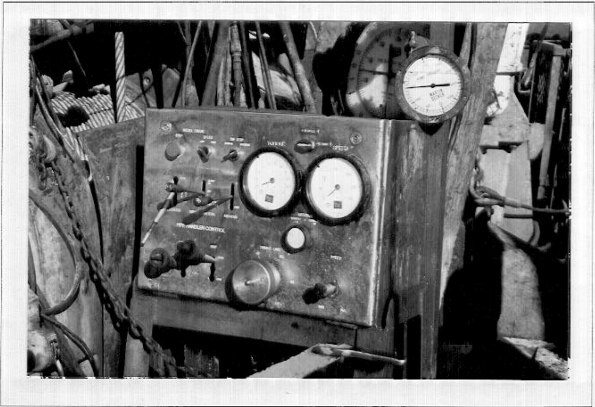
Driller's Control Panel After Accident
