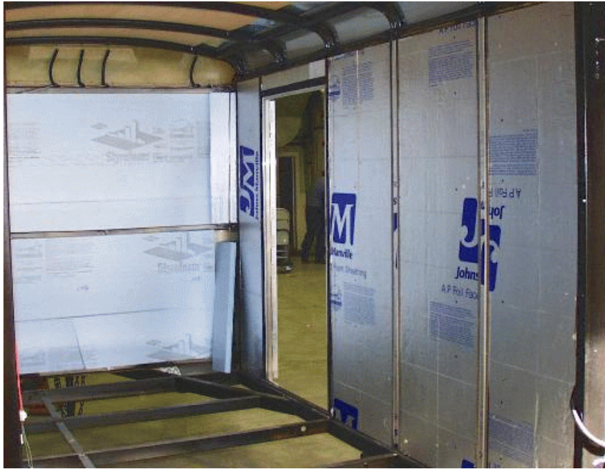
Figure 1. Inside of trailer with the floor removed and with insulation in the side and front walls.
