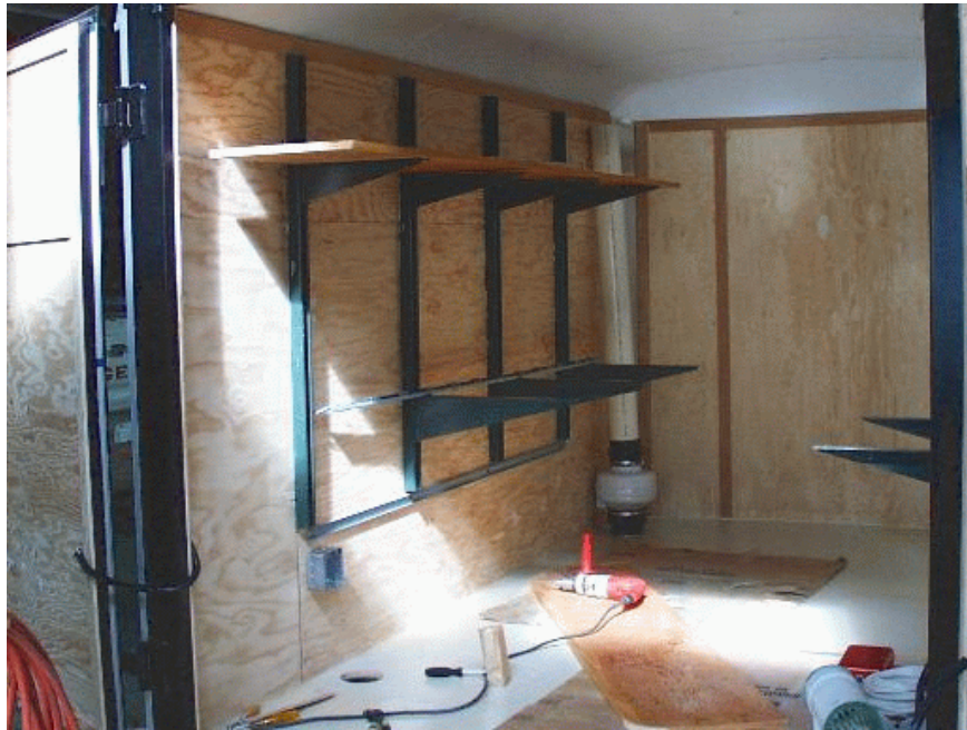
Figure 4. The insulation has been completed. Side panels have been reinstalled and ceiling has been fashioned and fit into place. Vent exhaust is located in the farthest corner. Fresh air inlet is located at the bottom right. Hole in the left side of floor is for AC and signal cable access.
