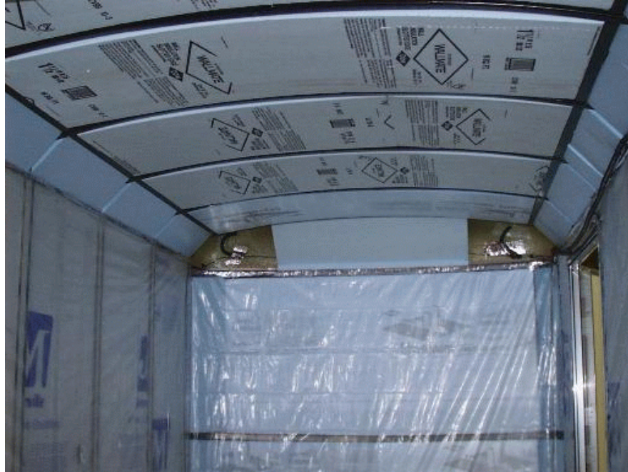
Figure 3. Side and floor insulation has been finished and the ceiling insulation is nearly completed.
