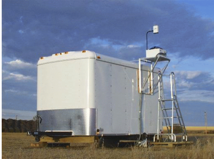
Figure 10. The completed installation. Note access steps to TSI.
