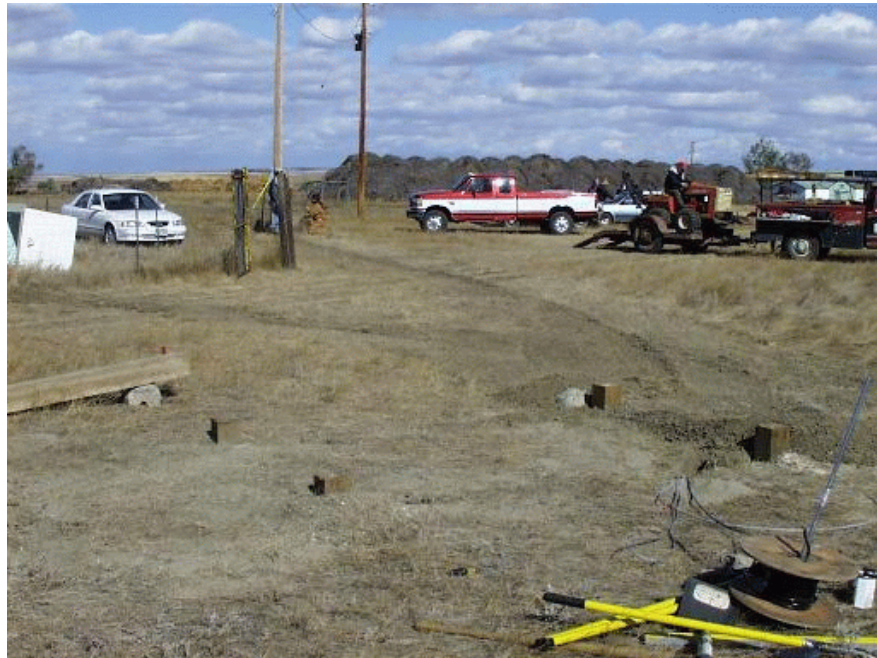
Figure 7. Four caissons in foreground. The filled trenches to the power pole and SURFRAD platform are visible.
