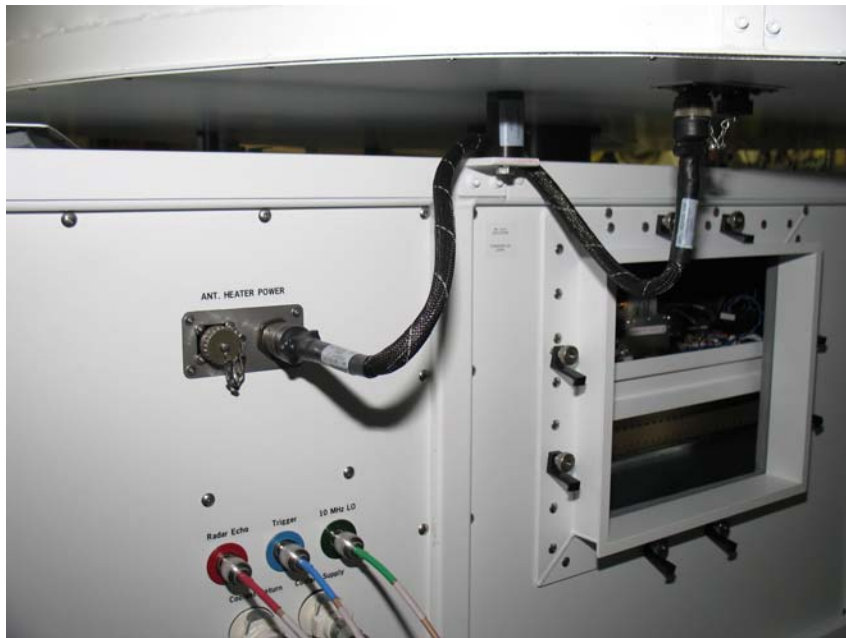
Figure 33. Antenna heater power connection.
