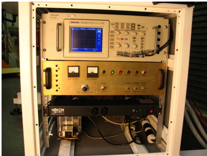
Figure 15. Digital oscilloscope, modulator power supply unit, and power strip mounted in RF Unit Environmental Enclosure.
