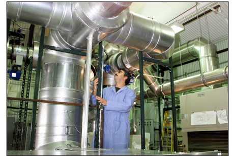
An ORNL researcher works in a maze of ductwork in the new Cooling, Heating, and Power Integration Laboratory.
