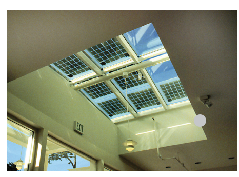
▲ The first model for demonstrating the integration of photovoltaics (PV) into a federal building is the sky-lighted entryway of the Thoreau Center for Sustainability at PRESIDIO NATIONAL PARK in SAN FRANCISCO, CALIFORNIA . Laminated to the skylight glass are PV cells that produce electricity while providing shading and day lighting.
