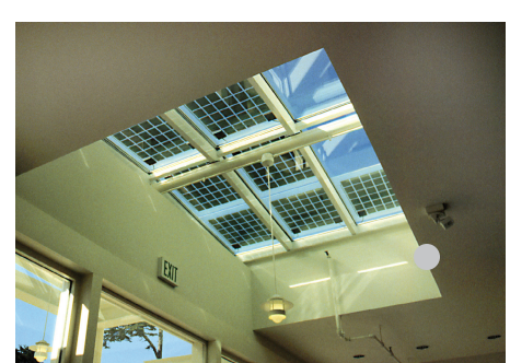
▲ The first model for demonstrating the integration of photovoltaics (PV) into a federal building is the sky-lighted entryway of the Thoreau Center for Sustainability at PRESIDIO NATIONAL PARK in SAN FRANCISCO, CALIFORNIA . Laminated to the skylight glass are PV cells that produce electricity while providing shading and day lighting.
