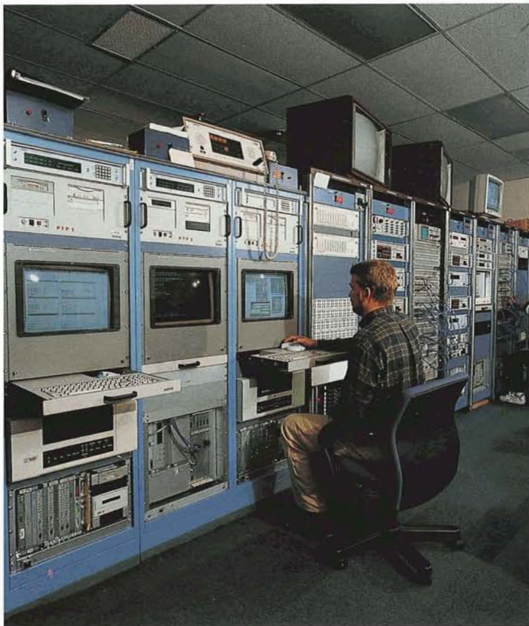
Avtec has provided telemetry hardware in support of NASA’s Communications Network (NASCOM). Shown are NASCOM boards at Goddard Space Flight Center’s Simulations Operations Center.
