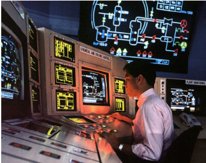
Figure 9. NUPLEX 80 Advanced Control Room design developed by ABB-Combustion Engineering
