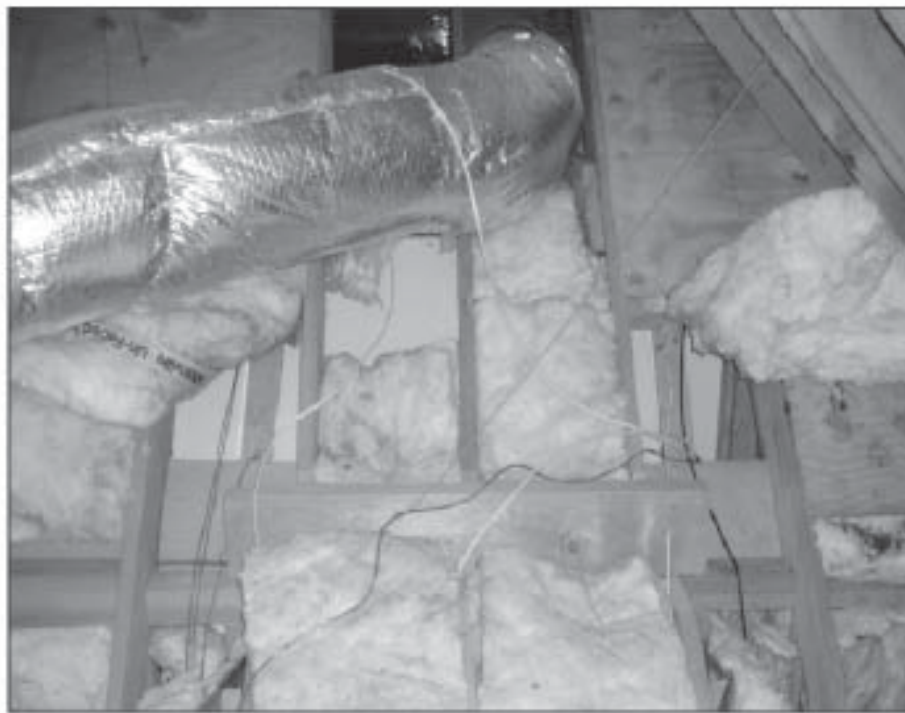
Figure 1a. BEFORE: Missing insulation on the sloped ceiling. Note that some of it is discolored, indicating an air leakage pathway.
