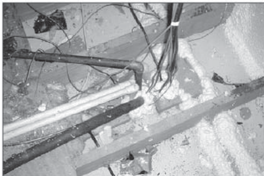
Figure 2: Plumbing, electrical, and other penetrations through the attic floor were sealed with spray foam prior to adding blown cellulose insulation. Old insulation was removed to reveal these holes.
