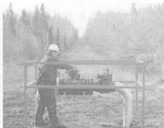
FIGURE 3.9-5 Natural Gas Control Valve
