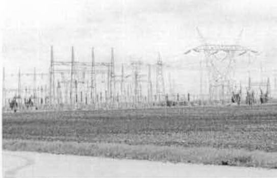
FIGURE 3.9-4 Transmission Lines Leaving Substation
