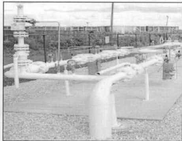
Typical natural gas city gate
