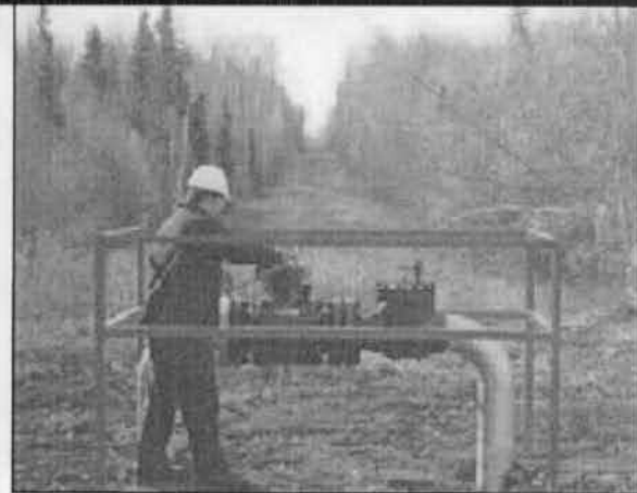
Natural gas control valve (note vegetation clearing that distinguishes pipeline location)
