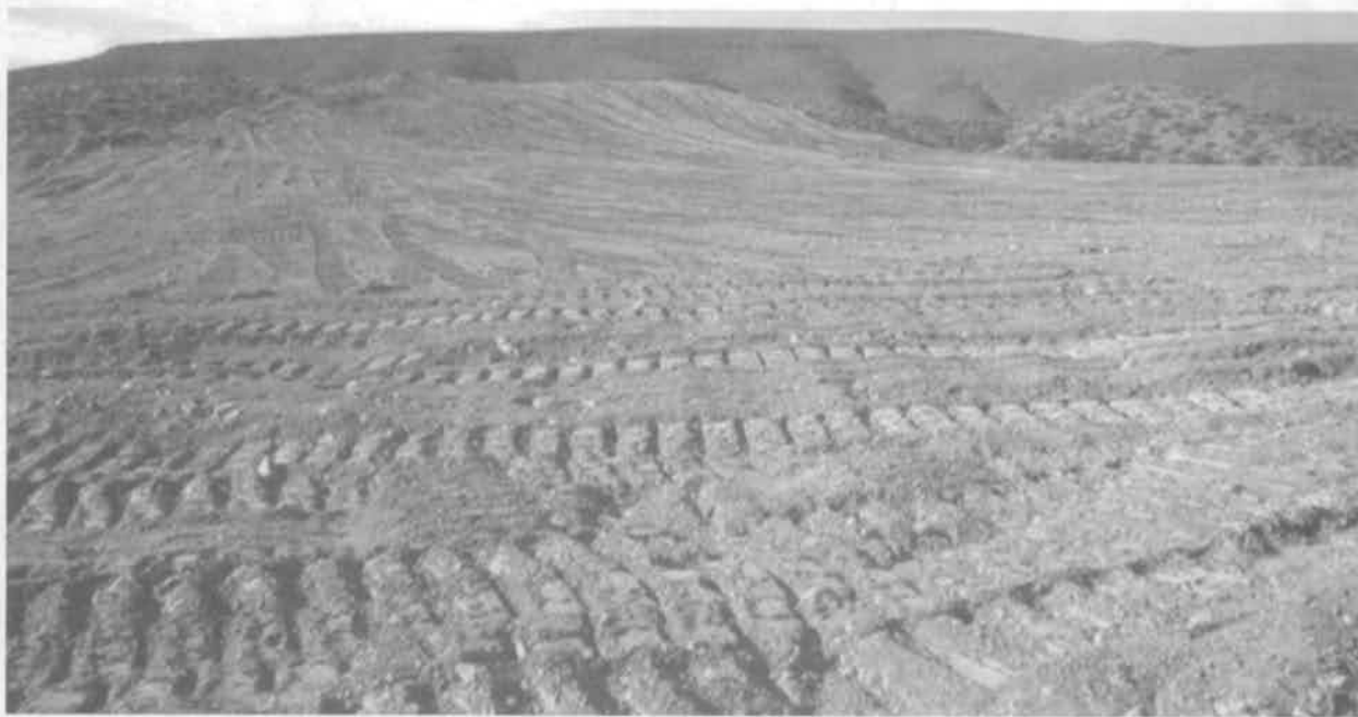
Figure 4-3. Decommissioned borrow area that has been recontoured prior to seeding and mulching.
