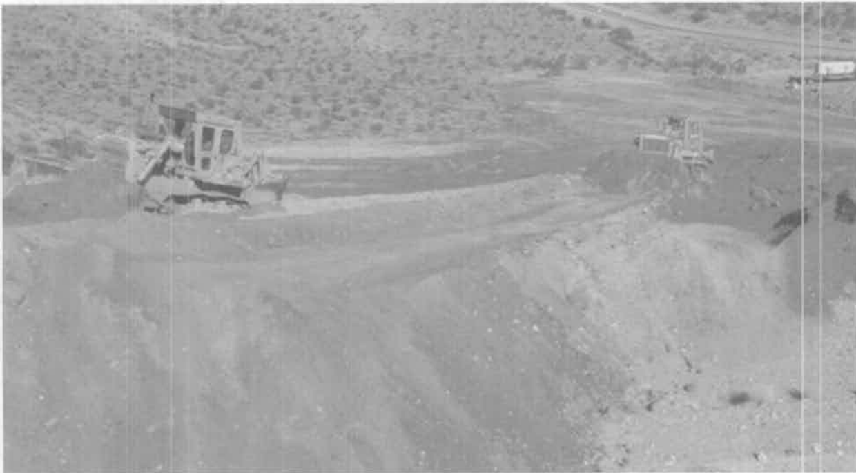
Figure 4-2. Fill material is spread and contoured on the site of a decommissioned borrow area.
