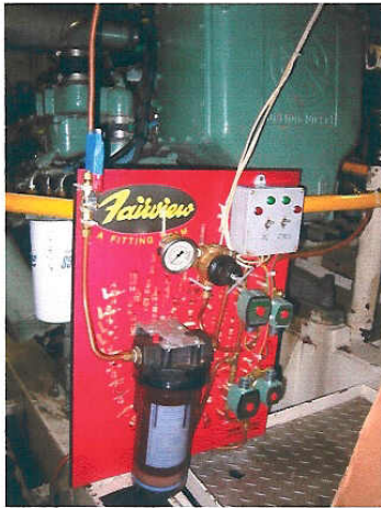
Water Injection Controls
