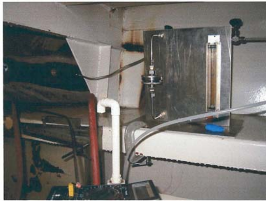
Particulate Trap and Filter/Dryer
