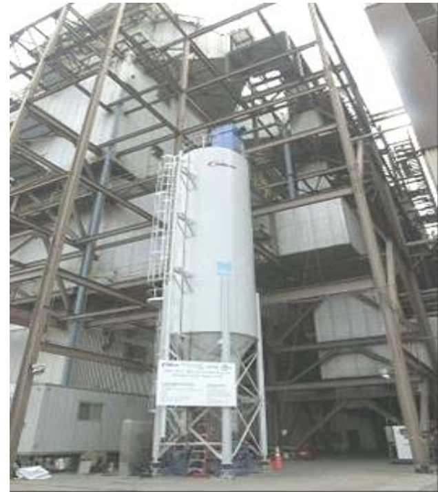
Activated Carbon Storage Silo
