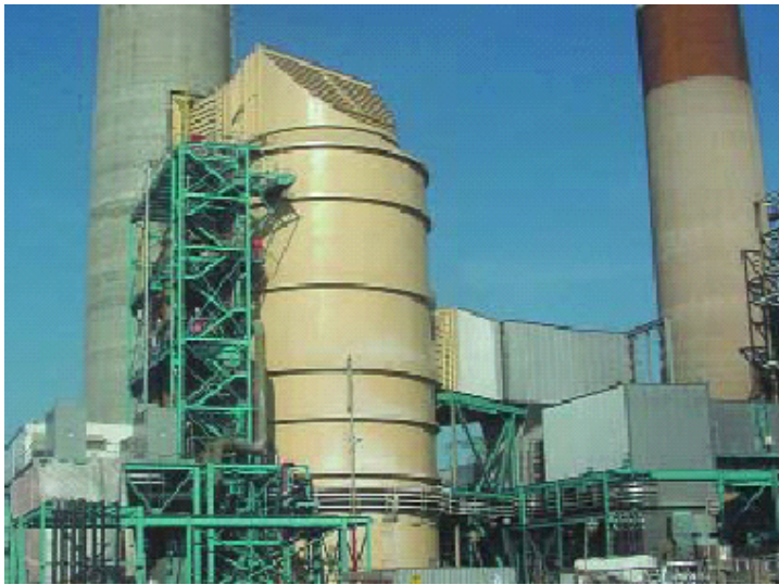
Wet FGD Scrubber
