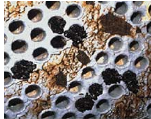
Intake Grate Partially Blocked by Zebra Mussels
