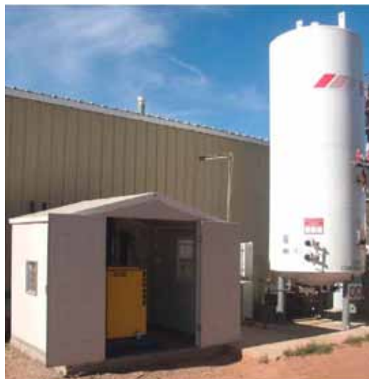
Figure 2. Compressors and Carbon Dioxide Unit at WRI
