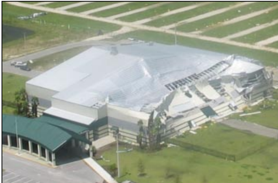
As it crossed Florida, Hurricane Charley badly damaged even such substantial structures as the Turner Agri-Civic Center in Arcadia, where 1,200 people sought shelter. There were 12 injuries at the center, but no deaths.
