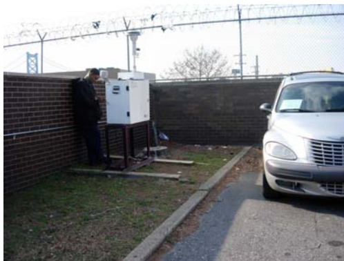
Figure 29 - Ground Level FAB Monitoring Station Picture
