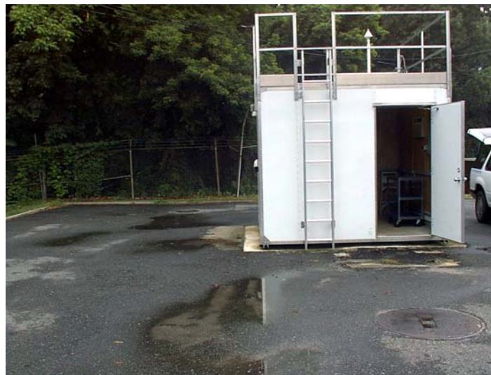
Figure 5 - Ground Level ROX Monitoring Station Picture
