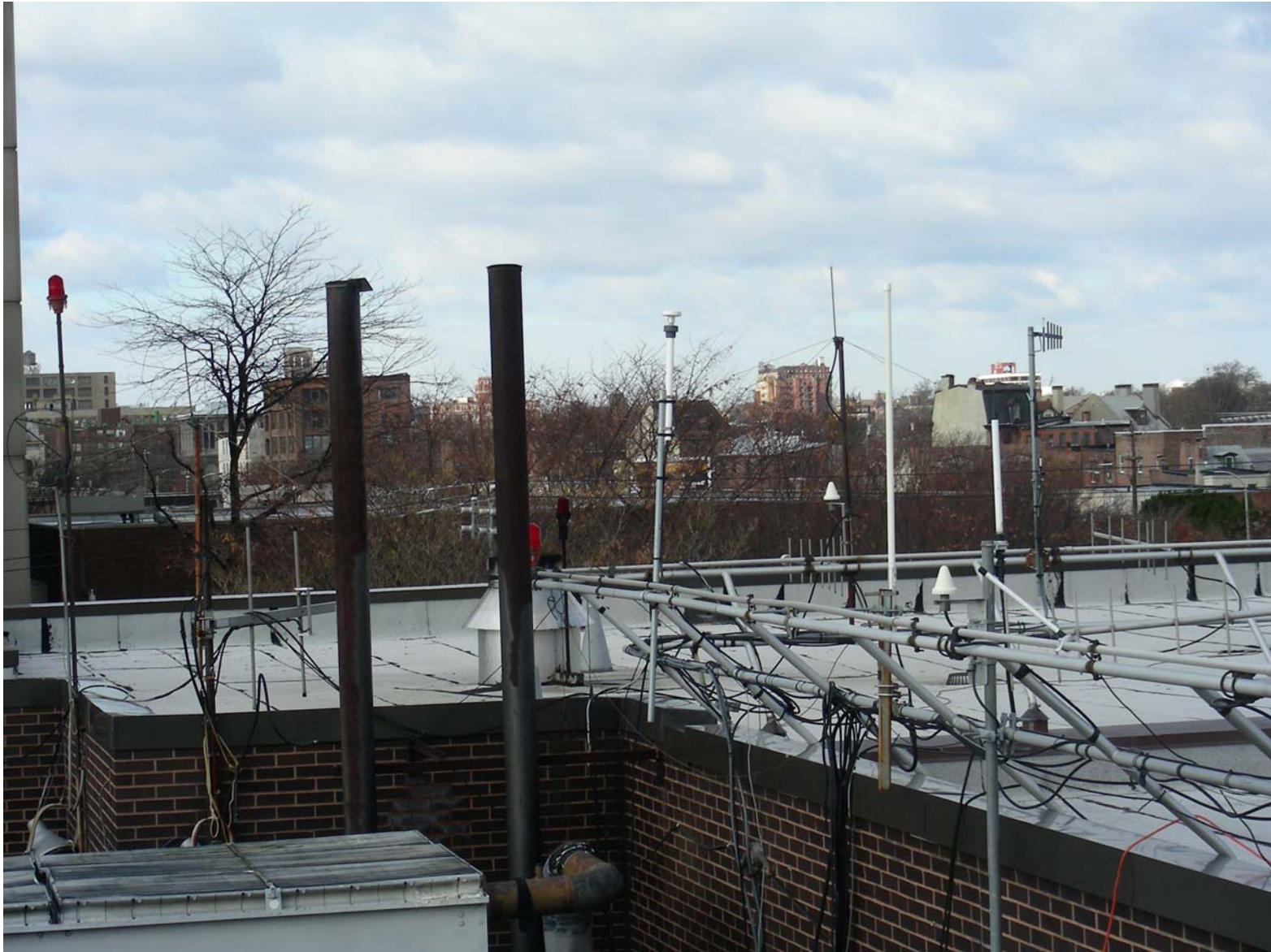
View of two emergency diesel exhausts and the top of the mechanical area.
