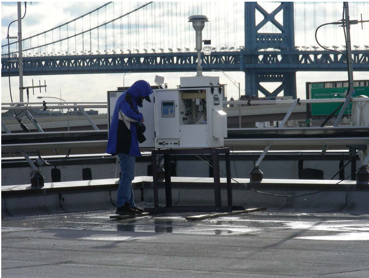
Fire Dept. HQ PM 2.5 Sampler on roof.
