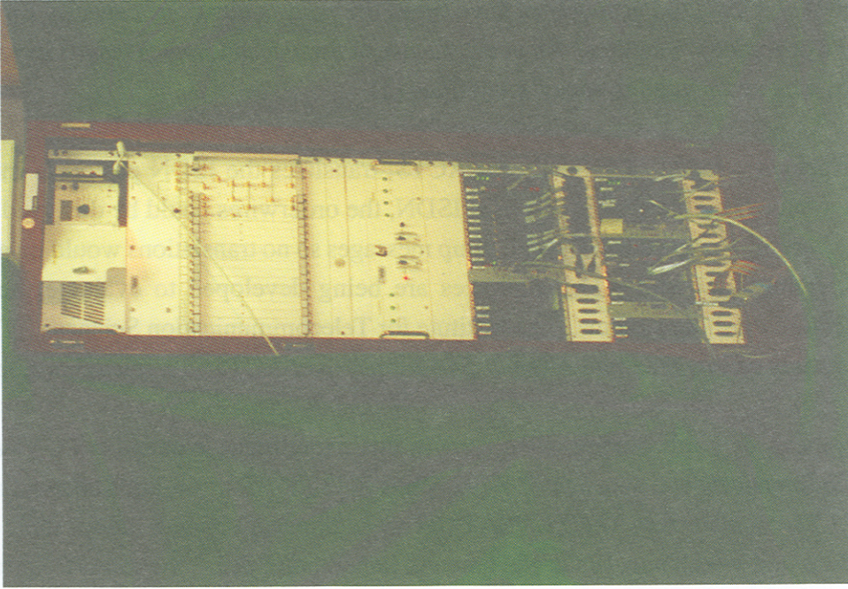
Figure 2. T1-VSAT indoor unit.
