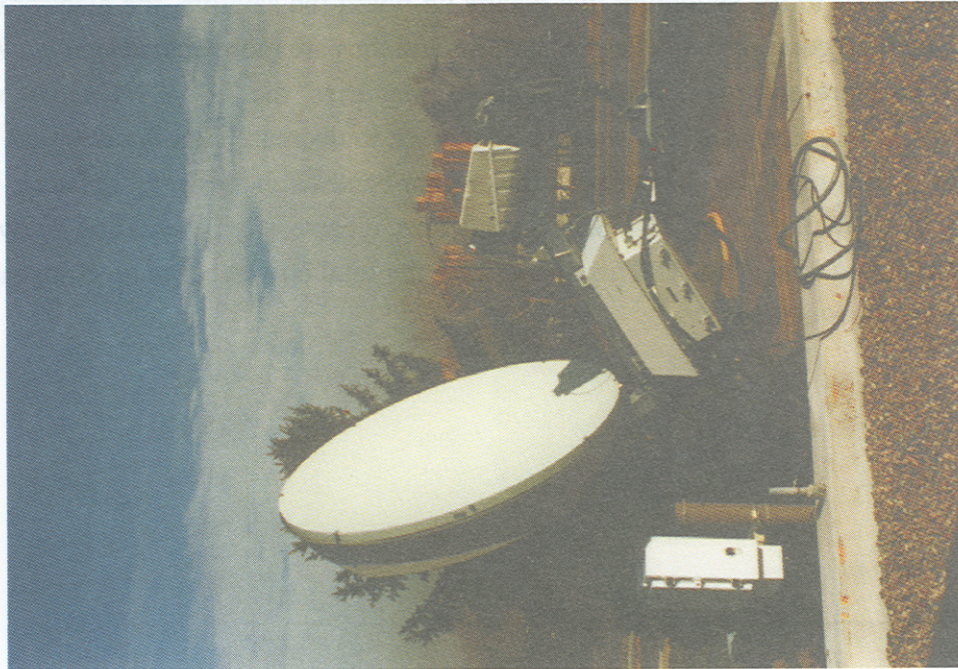
Figure 1. T1-VSAT outdoor unit.
