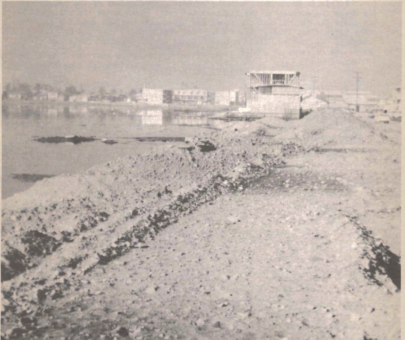
Land fills to hold apartment complexes are among the many current threats to light-footed rail habitat. This one is at Tijuana Estuary, California. Photo by S. Wilbur.
