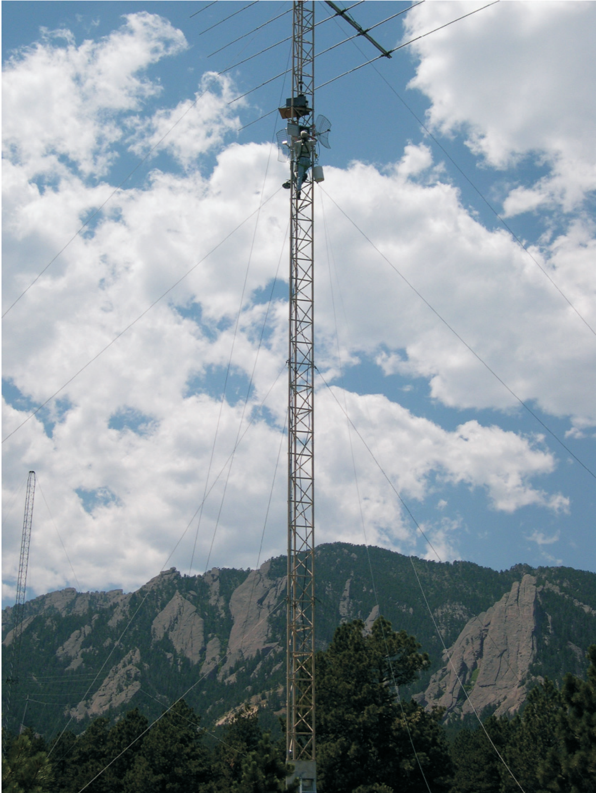
Telecommunications Engineering, Analysis, and Modeling Division engineer installing an antenna at the Green Mountain Mesa field site, part of the short & long range wireless test links (photograph by C. Redding).
