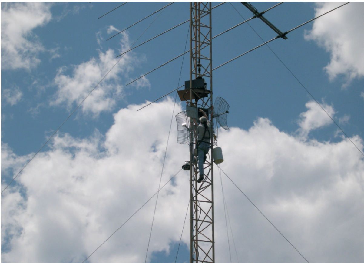
ITS engineer installing an antenna at the Green Mountain Mesa field site (photograph by C. Redding).
