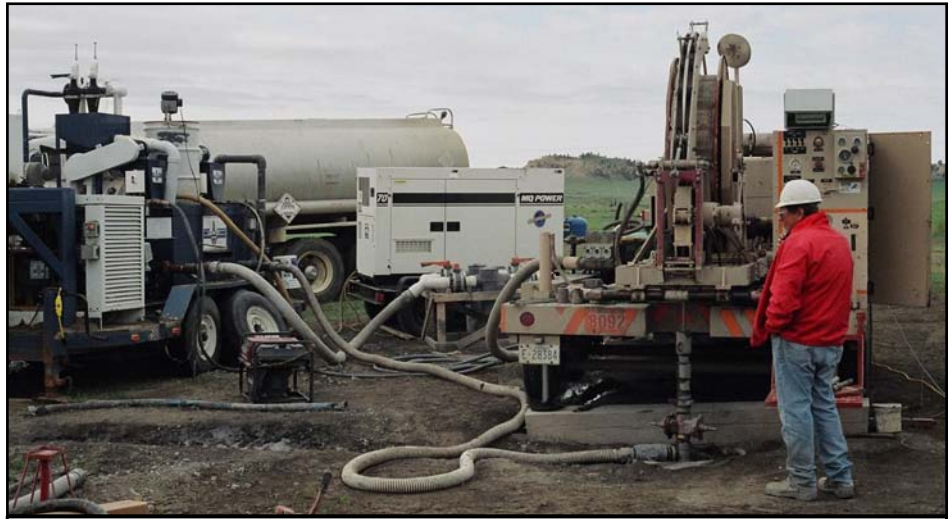
LANL microdrilling at the RMOTC-operated Teapot Dome Field at NPR No. 3. The microdrilling rig includes the coiled tubing drilling unit on the right, mud cleaning system on the left, and the RMOTC drilling-water truck in the center.
