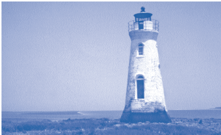
Work teams rebuild exterior walls of the historic Cockspur Island Lighthouse at Fort Pulaski National Monument.
