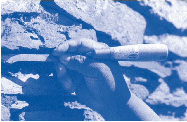
NPS worker repairs crumbling mortar of ancient walls at Arizona's Wupatki National Monument as part of the NPS Vanishing Treasures Initiative.
