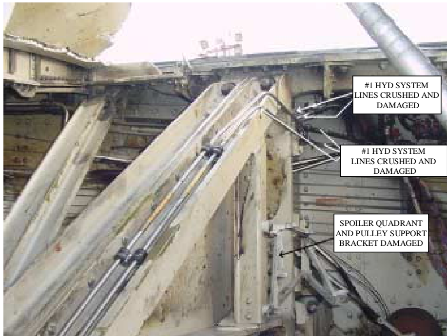
Figure 1 –Damaged #1 Hydraulic System Lines
