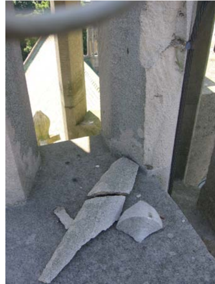
Figure 2.2: Stone spall at mechanical anchors
