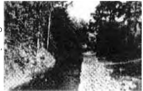
USE OF GRANITE TO CONTROL SOIL EROSION ALONG PEAVINE CREEK. GRANITE USED AS “RIP RAP” IN ADDRESSING BANKSIDE EROSION IS EFFECTIVE, BUT MORE AESTHETICALLY- PLEASING MATERIALS CAN BE USED WITH THE SAME RESULT. NATIVE ROCK MATERIALS INSTEAD OF GRANITE BLEND
