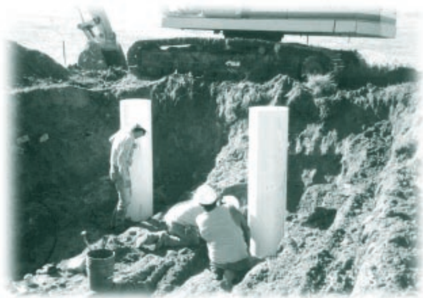
Construction of Mni Wiconi rural water project in South Dakota (photo by Reclamation).
