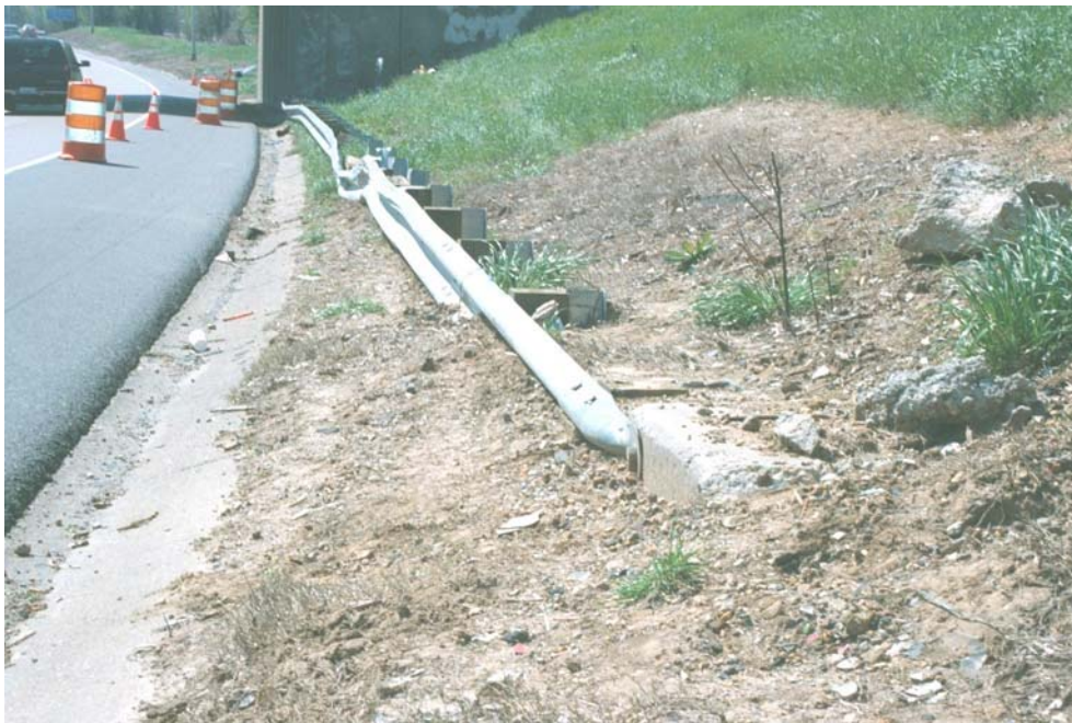
Guardrail and terminal unit at accident site.
