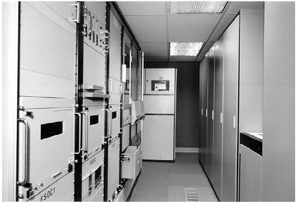
▲ Figure 1. Equipment racks, part of the Integrated Polar Acquisition and Control (IPACS) that will be used to control satellites in the Defense Department's Defense Meteorological Satellite Program (DMSP), were recently installed in NOAA's Satellite Operations Control Center in Suitland, MD.
