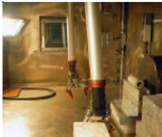
Hotbox facility (interior) at the MIT Reactor Laboratory
