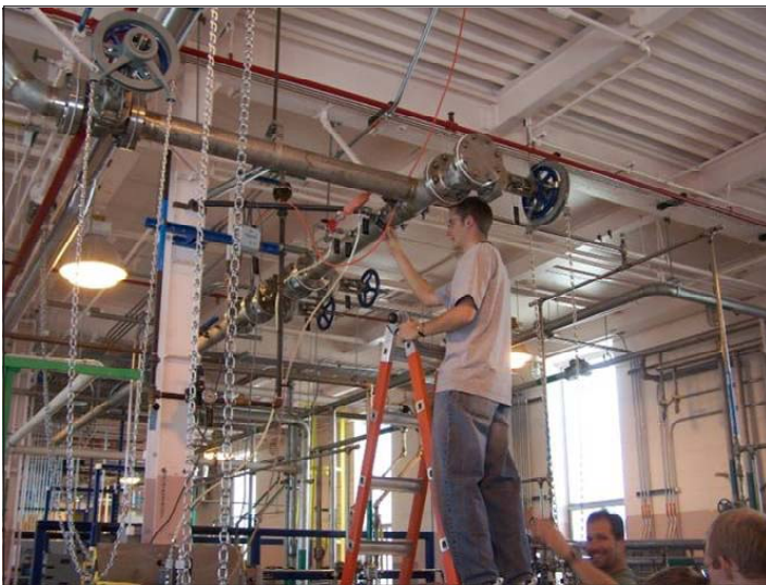
Caleb Robison working at the TRA-608 demineralizer building that provides high purity water to the Advanced Test Reactor at the Idaho National Laboratory.
