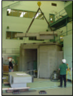
Concrete is poured for the new Neutron Radiography Facility at Oregon State
