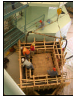
Section 4 of the roof for the Neutron Radiography Facility at Oregon State is lowered into place
