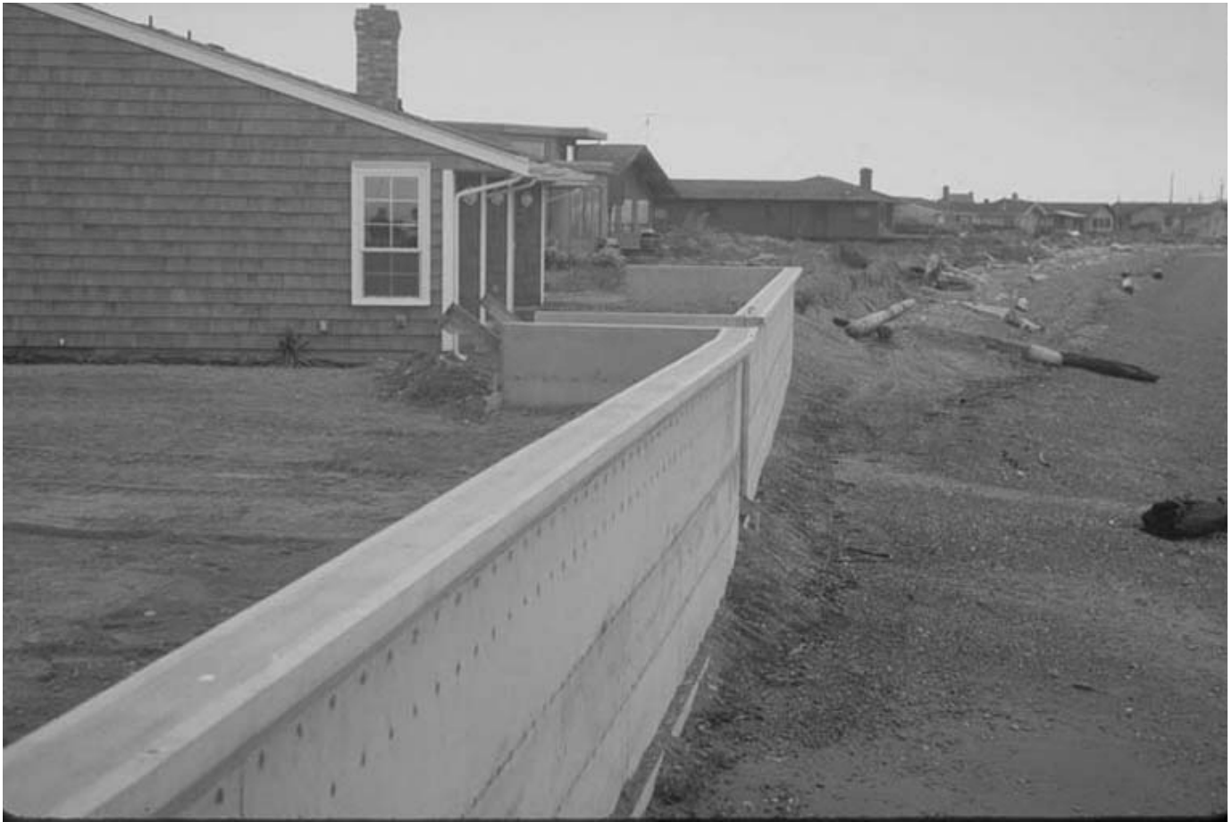
▲ Figure 2. Bulkhead-induced erosion, a result of failing to take natural processes of shoreline erosion and sedimentation into effect.
