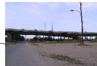
Bridge ramps at Poplar Point: a confusing sequence of ramp configu- rations from the Frederick Douglass Bridge
