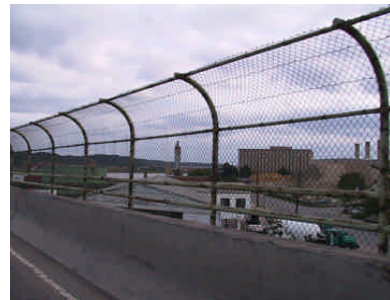
Pedestrian walkway on Frederick Douglass Bridge: an aging structure designed with dangerously narrow pedestrian access
