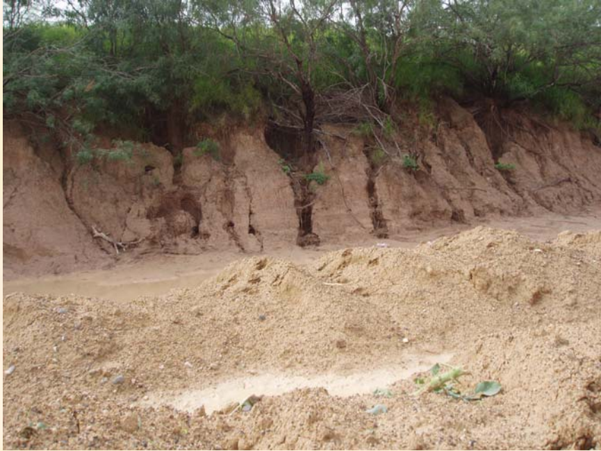
Embankment Erosion at Morillo Drain Encasement Site
