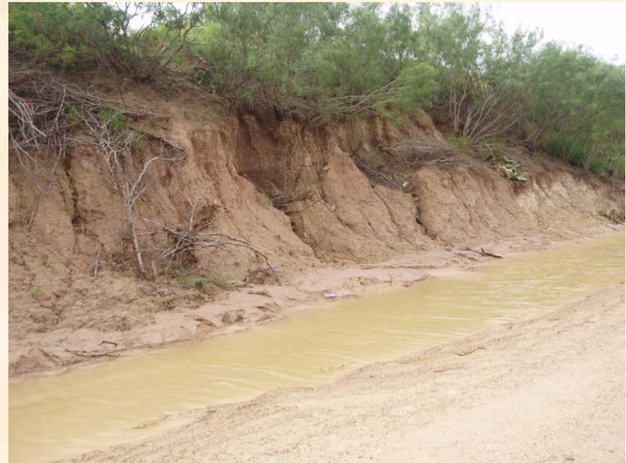
Embankment Erosion at Morillo Drain Encasement Site
