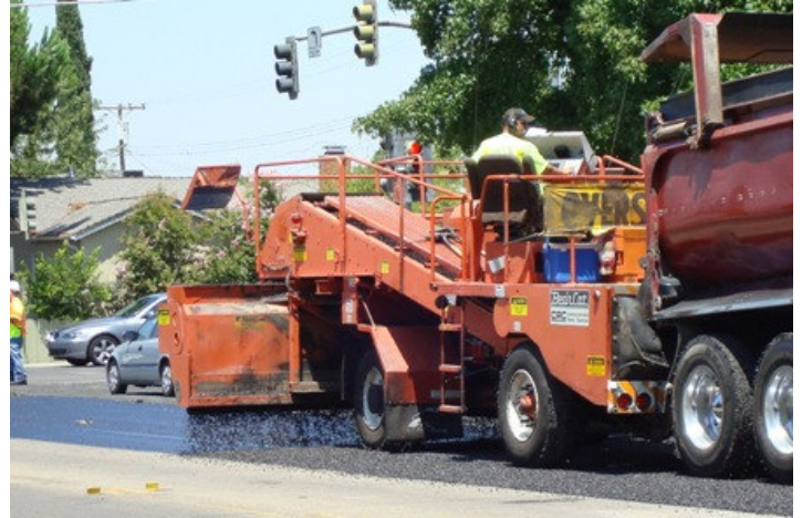
Workers place a layer of coated gravel onto a mixture of oil and rubber on Ham Lane as part of Lodi's recent road maintenance project.
