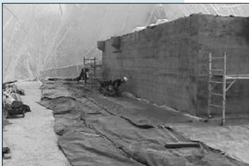
Concrete foundation to support the coal-diesel engine and generator being poured inside heated tent during subfreezing weather in Fairbanks.
