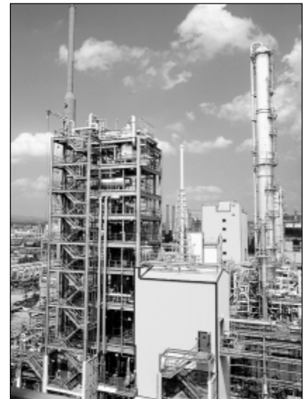
The LPMEOH™ plant applies new technology to produce methanol from coal-derived synthesis gas.
