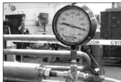
Gauge measures water pressure and possible leaks in loop system prior to installation in boiler
