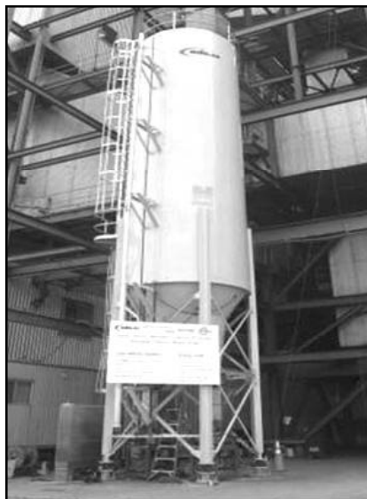
Storage silo for activated carbon
