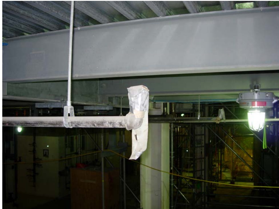
Figure 6: Paper taped covered sprinkler heads
