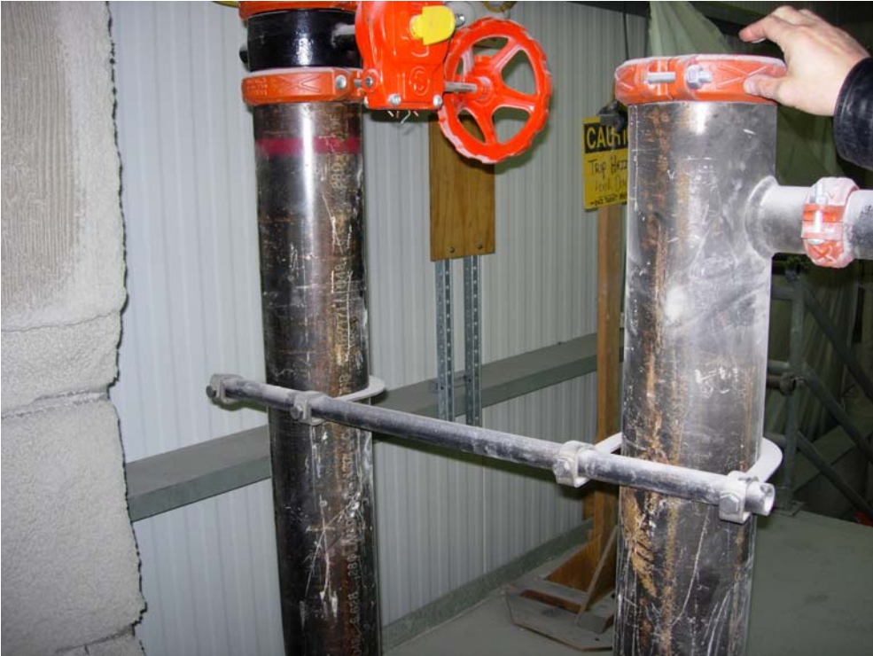
Figure 4: Sway bracing not connected to structure but other sprinkler piping +48 foot elevation
