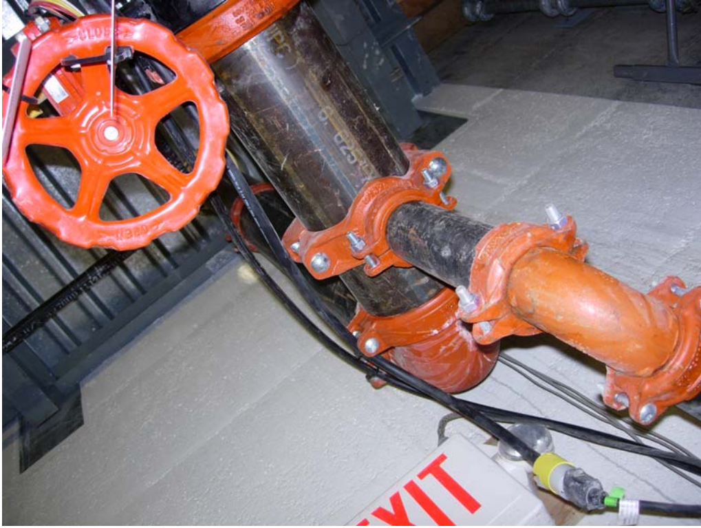
Figure 10: Mechanical T's missing 'coupons'
