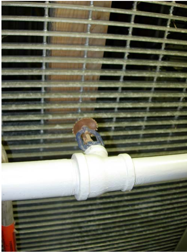
Figure 7: Incorrect installed heads under mezzanine grates & missing head guards in areas subject to physical damage
