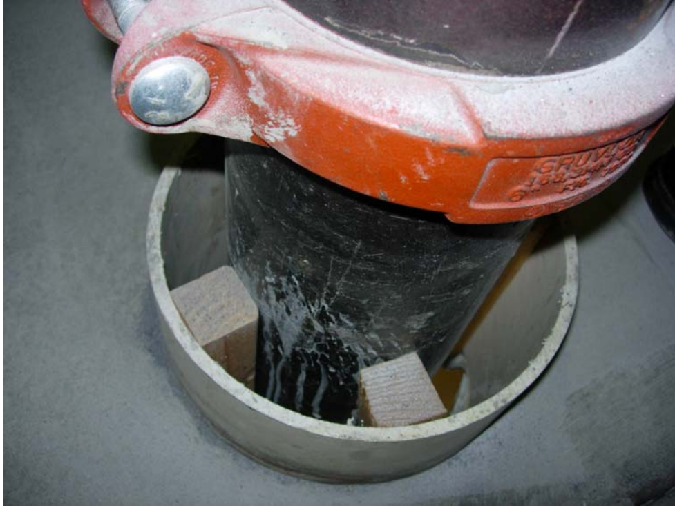
Figure 5: Combustible wedges left in riser floor sleeves
