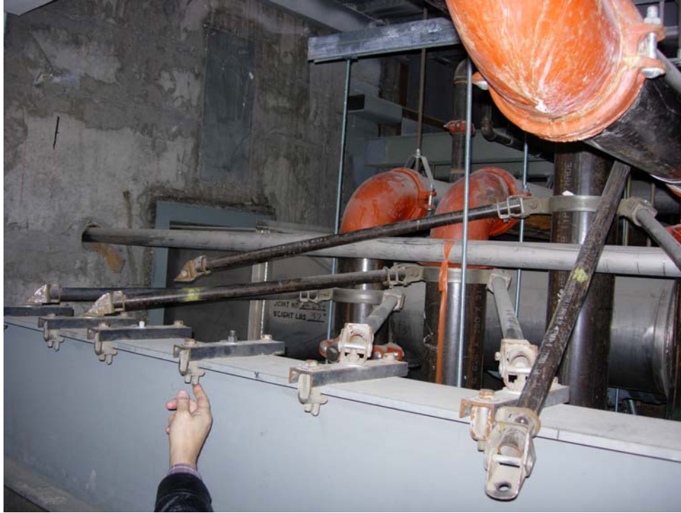
Figure 1: Disconnected Sway Bracing at -21 foot elevation
