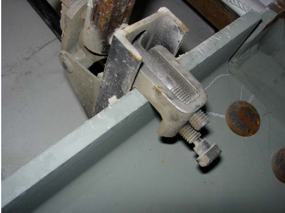
Figure 3: Improperly torqued cone point set bolt on “TOLCO” sway brace at N.E. stairwell 28 foot elevation
