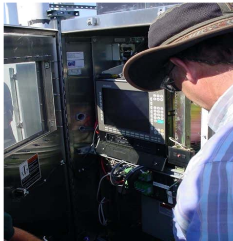
Inside PLC Enclosure 110
