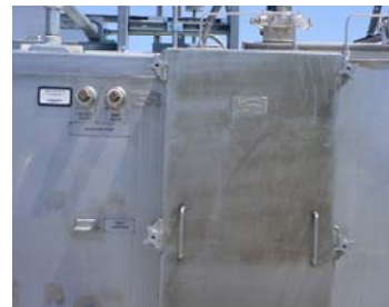
AN "B" Train Missing Labels
