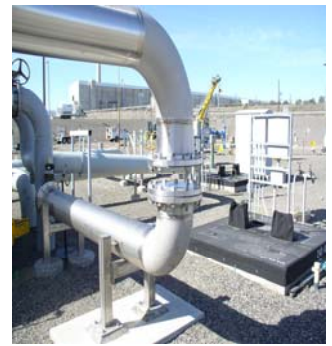
AW Isolation Point
