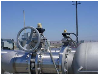
AN Demister Valves, One Open and One Closed
