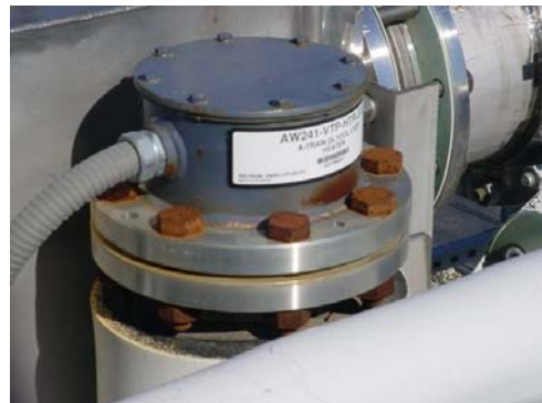
AW Rusted Bolts on Glycol Heater
