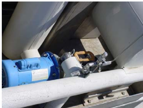
AN Glycol Pump and Valve Open
