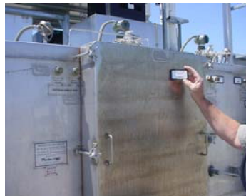
AN "A" Train Missing Labels
