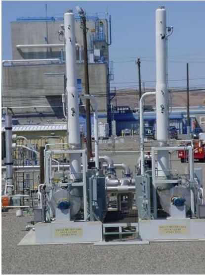
AW Exhauster from the South
