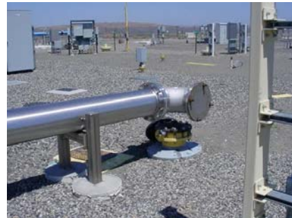
AN Isolation Point
