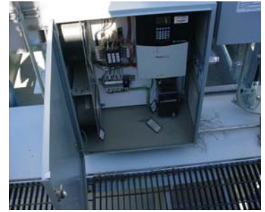
Dust in Variable Frequency Drive Enclosure AW
