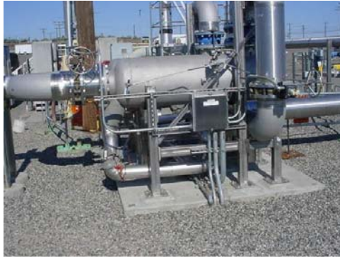
AW Demister Drains Closed
