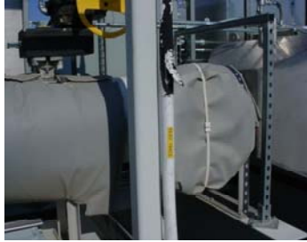
AW Torn Insulation
