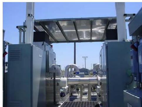
AN Sun Shade Over Skid Panels
