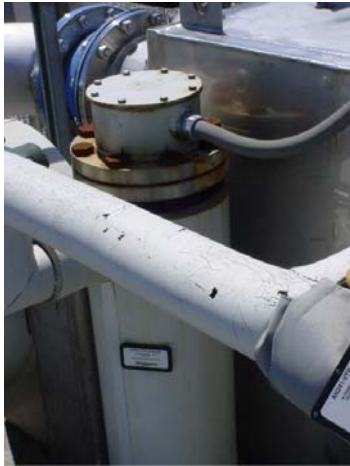
AN Glycol Heater Rusted Bolts
