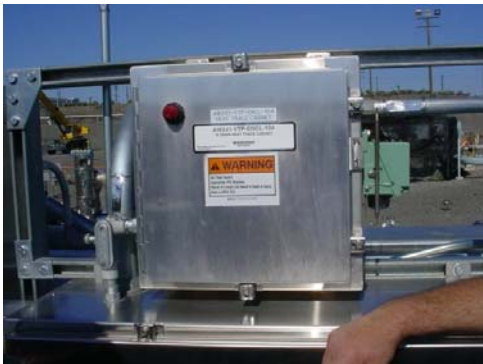
AW Heat Trace Enclosure 104
