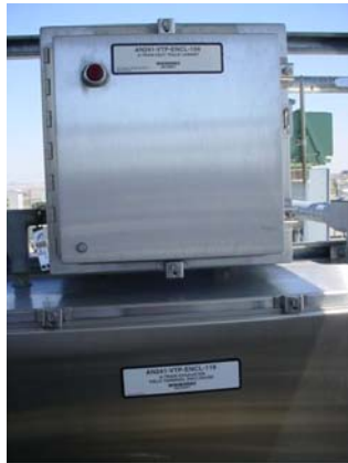
AN Heat Trace Cabinet 104
