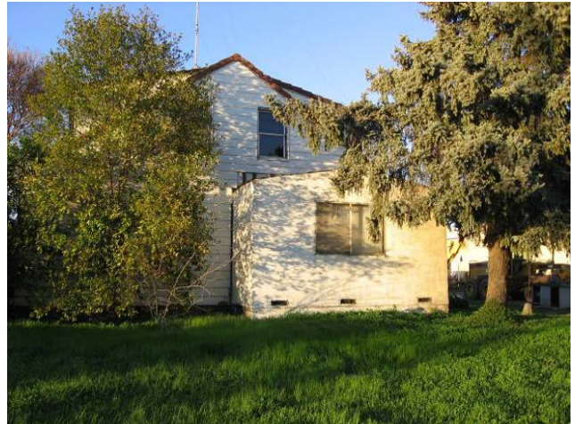
Photo A1 Damaged exterior walls and roof, and a room addition that is likely unpermitted.
