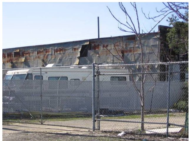
Photo A3 Large portions of the exterior wall surface are missing.
