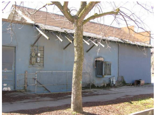
Photo A2 Damaged exterior walls and roof with large portions of the roofing material missing. This building is vacant.
