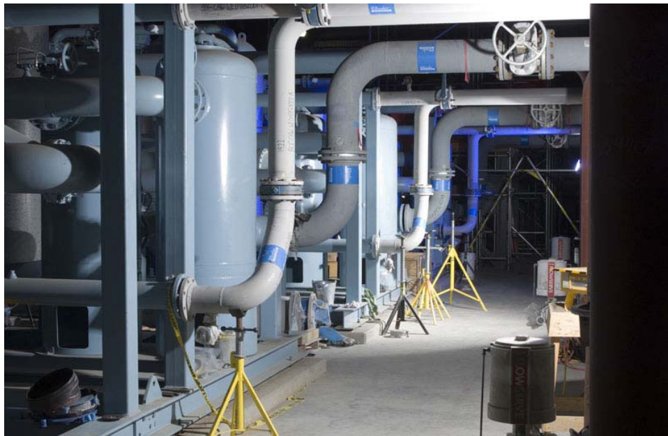
Figure 3. Piping in the Chiller Compressor Plant
