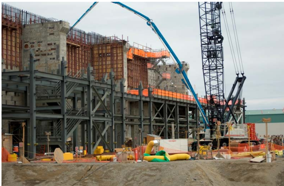
Figure 5. Pretreatment Facility – South Side
