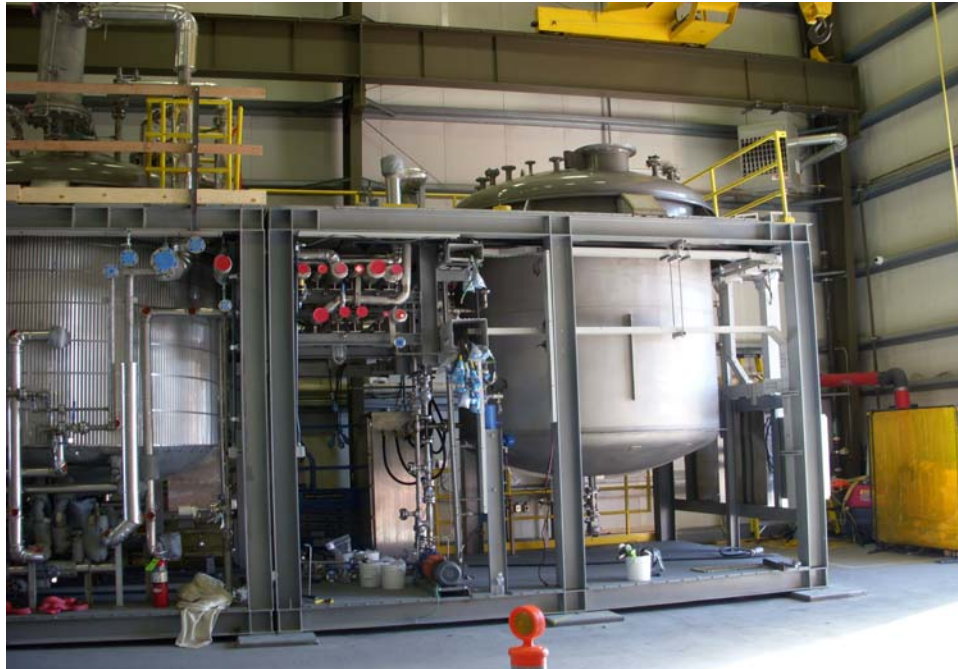
Figure 6. Pretreatment Engineering Platform (Evaporator Vessel)
