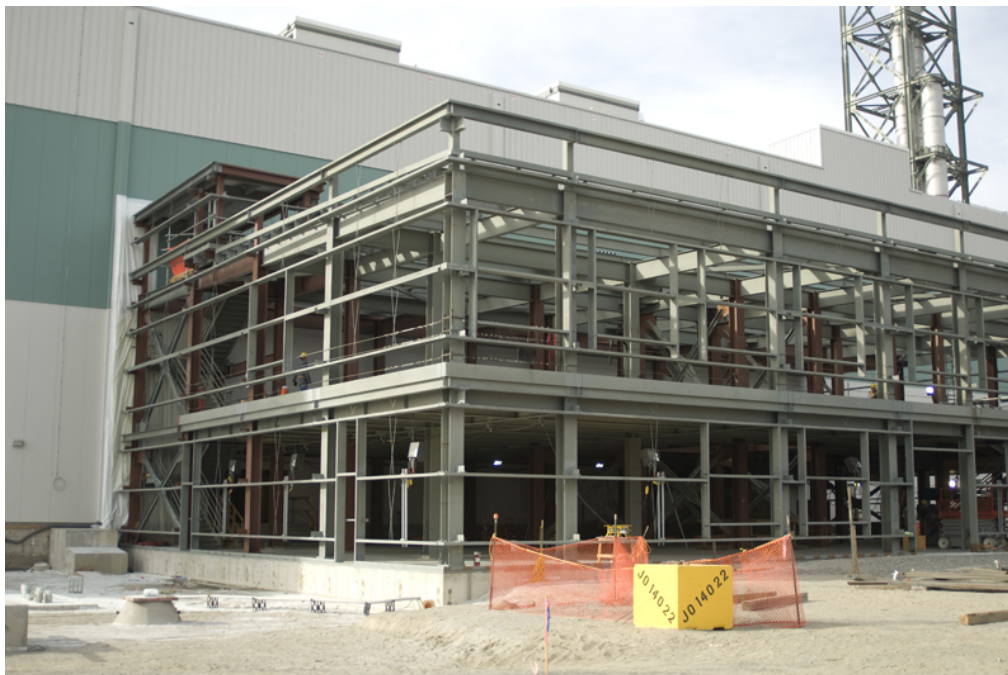
Figure 3. LAW Control Room and Office Annex
