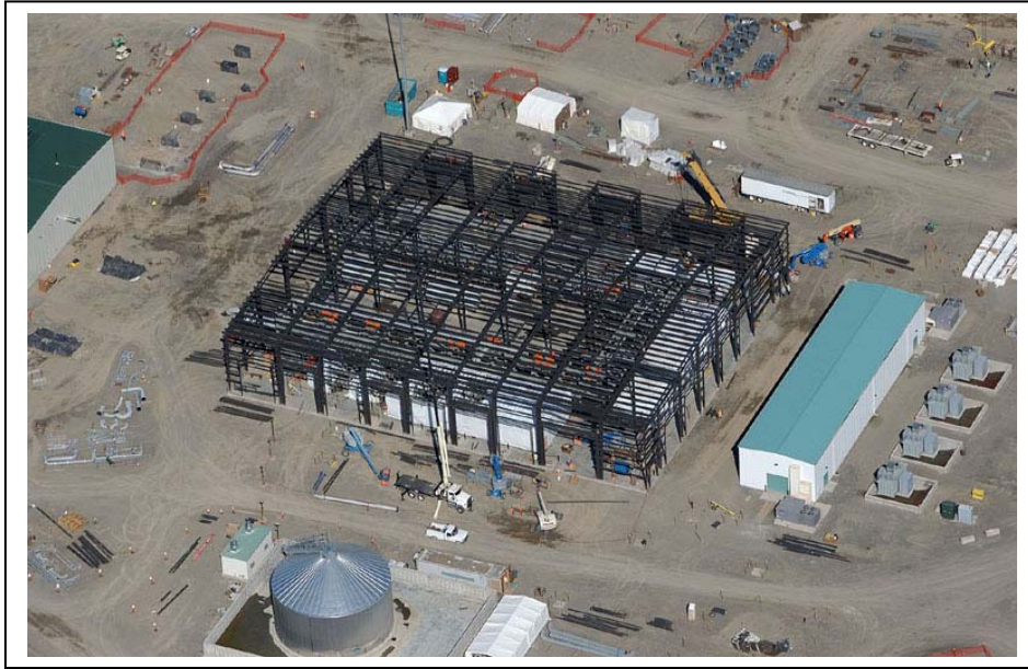
Figure 4. Chiller Compressor Plant
