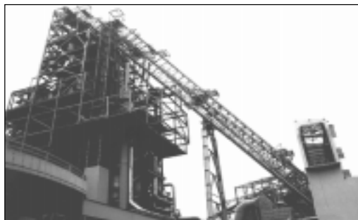
Expansion of the existing iron-making capacity at the POSCO Pohang Works (Republic of Korea) using COREX® technology.
