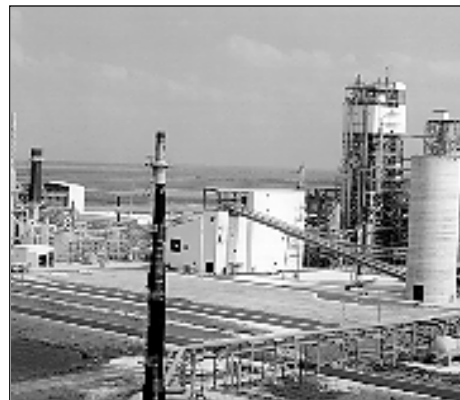
Aerial view shows Tampa Electric's 250-MWe greenfield IGCC unit at the Polk Power Station in Lakeland, FL.
