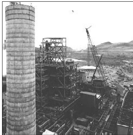
Northwest view of Gasifier Island with coal storage dome in background.
