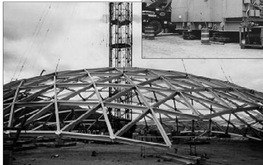
The erection of a novel geodesic dome for enclosed storage of feed coal in the Piñon Pine Project.
