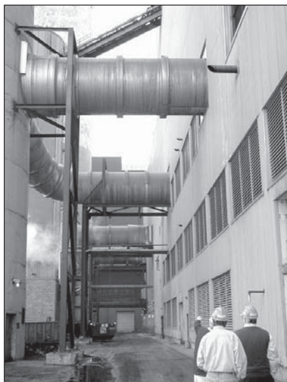
Ductwork at Presque Isle plant
