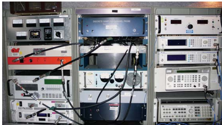
Figure 1. Interior view of the ITS propagation measurement transmitter van (photograph by F.H. Sanders).
