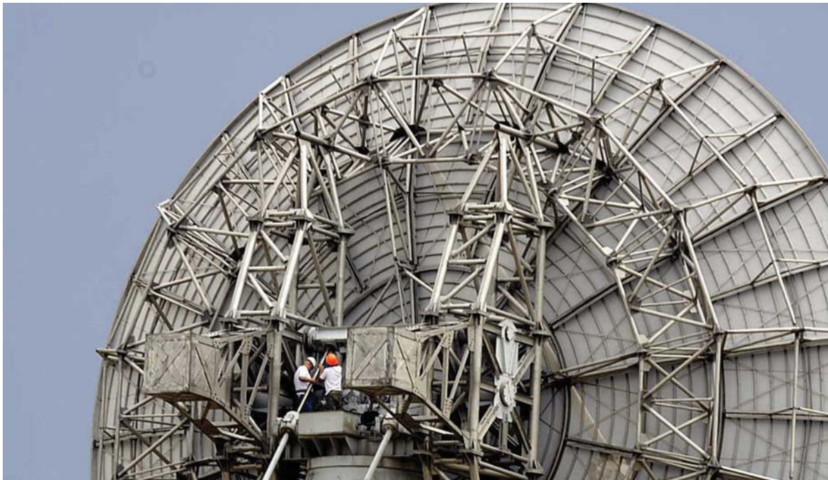
DSES group replacing the jack screw boots on the main dish drive mechanism of one of the 18.3-meter parabolic dish antennas at the Table Mountain field site (photograph by J.W. Allen).
